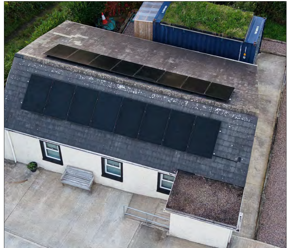
The new solar panels on Annaghmore Orange Hall. Picture by John Whyte.
